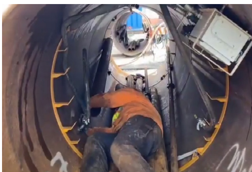
A worker inspects a portion of the new sewer main casing before installation
