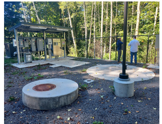
New Pump Station 31 is an in-ground station at 7105 Clover Blossom Lane
