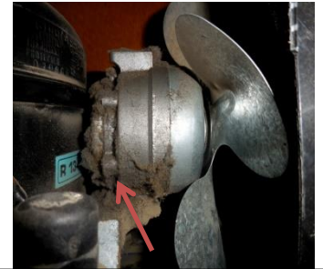
Dusty compressor! Needs to be vacuumed.
